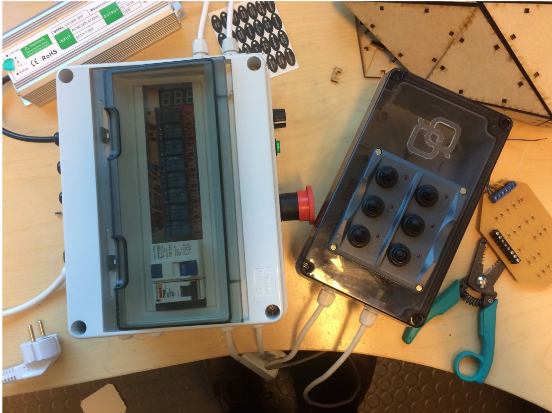
Fig. 39: Switch and Control Panels.
